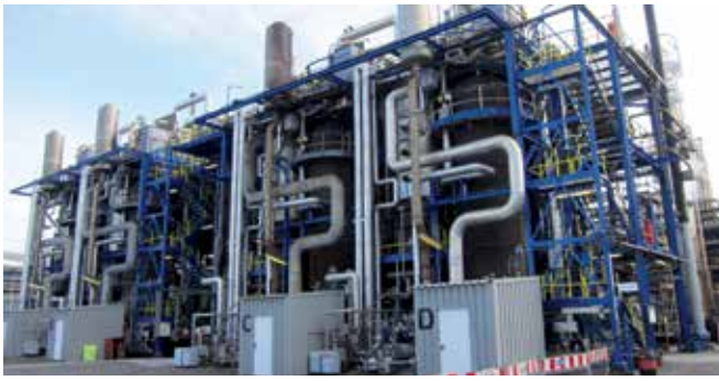
The four reactors of the POX-gasification plant at Yara Brunsbüttel
