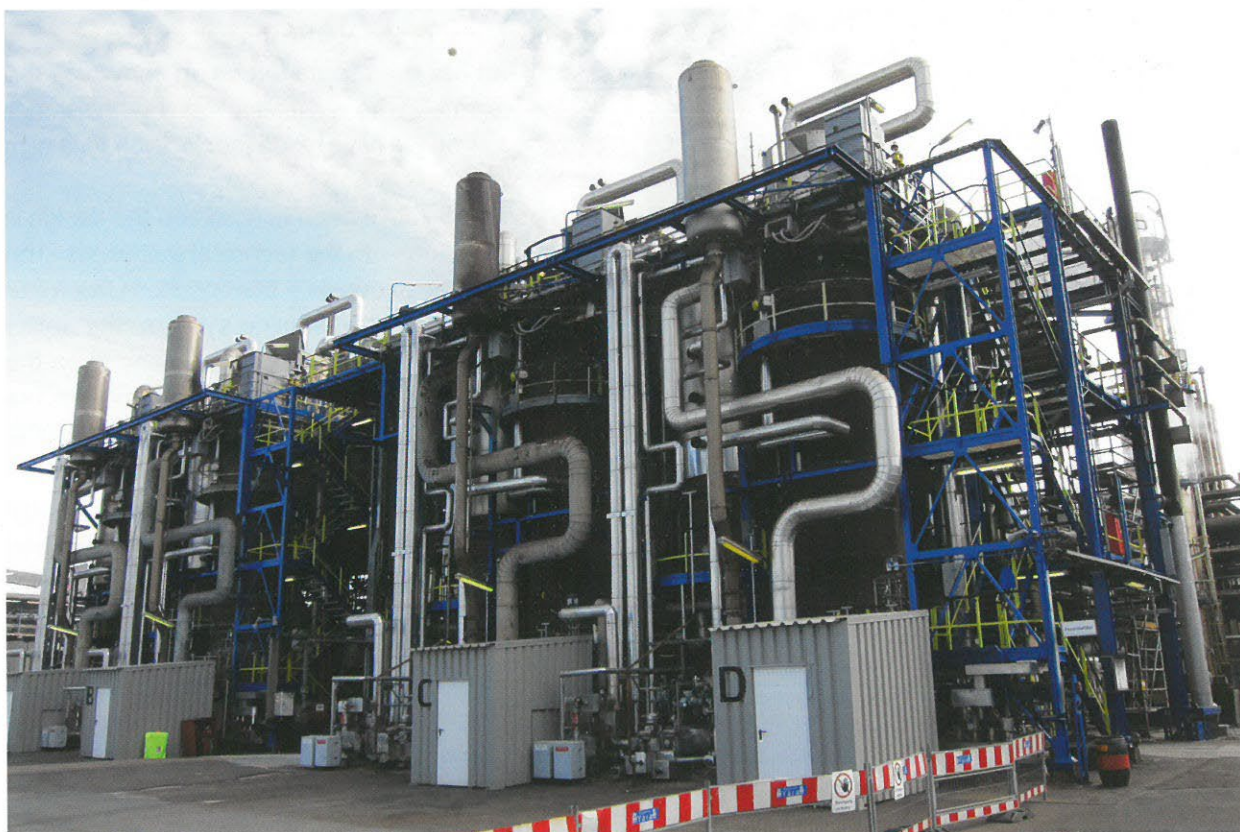
Figure 2: The four reactors of the POX-gasification plant at Yara Brunsbüttel, Germany.
