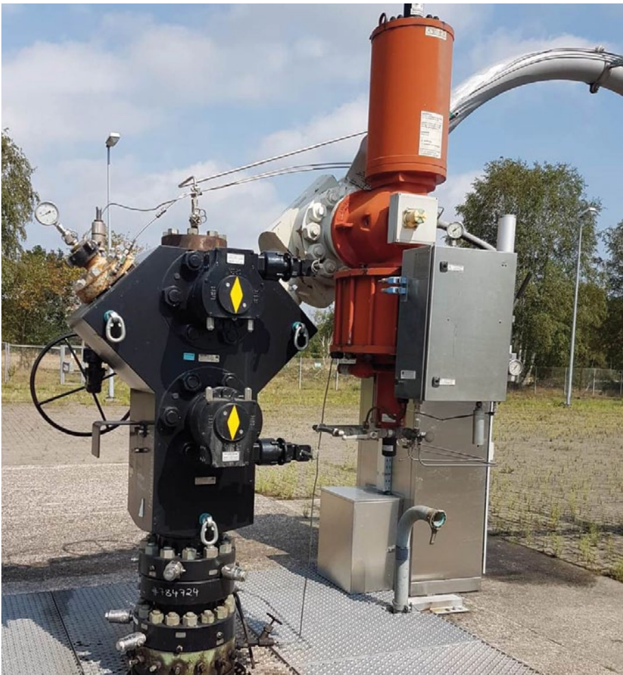
Fig. 1 Successful changeover: The X-Mas tree with ball valves and quick-acting shut-off valve is almost maintenance-free while used in gas production
