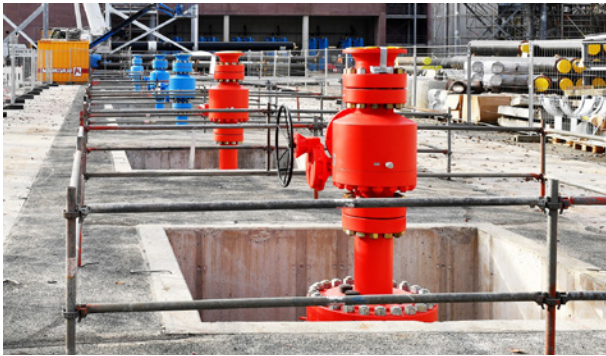
Image 2: At the largest German geothermal project by SWM (Munich public utilities), six Hartmann wellheads with ball valves provide a secure shut-off.
